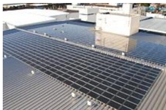
Solar power generation panel at Kumagaya Plant
