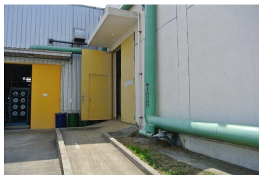
Steam pipes running inside the premises at Nikon Imaging (China) Co., Ltd
