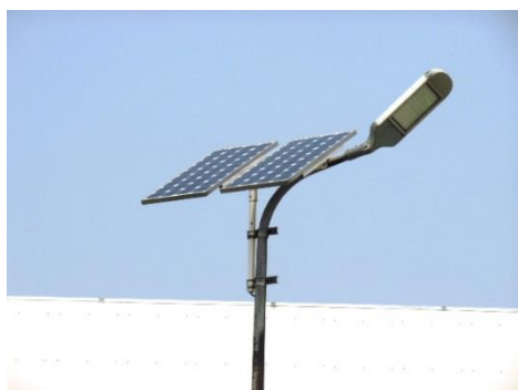
LED outdoor lighting with solar panel at Nikon Imaging (China) Co., Ltd.
