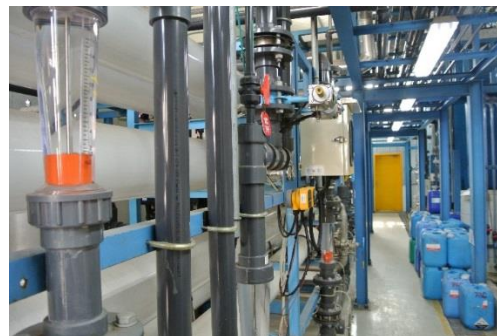
Reuse of concentrated water discharged from the RO water* purification process at Nikon Imaging (China) Co., Ltd.
