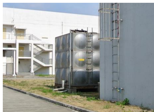
Concentrated water storage
